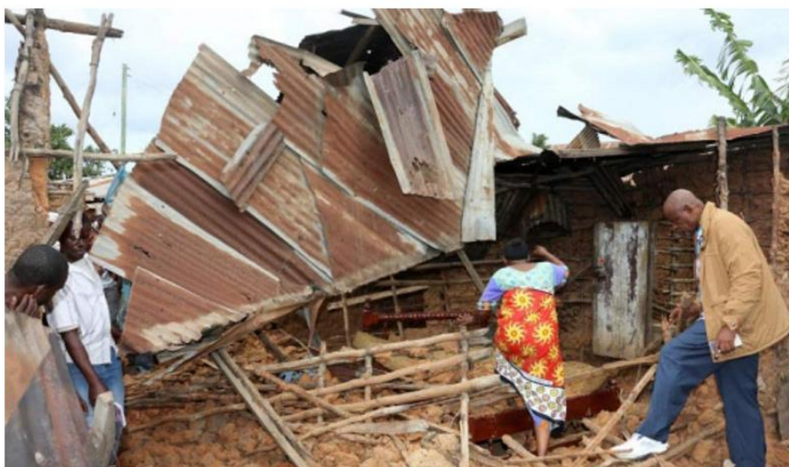
Picture 4: Wind damage to a school building
